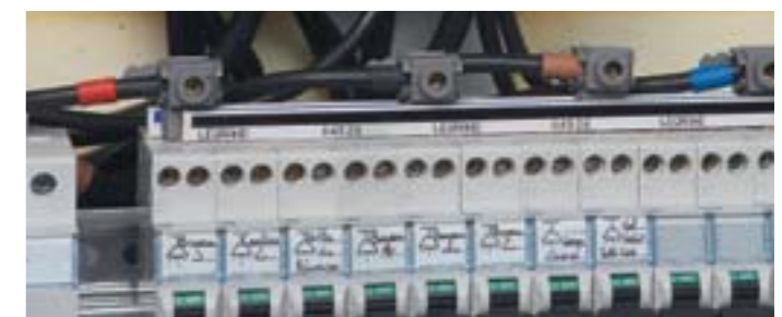
^ Distribution via supply busbars
